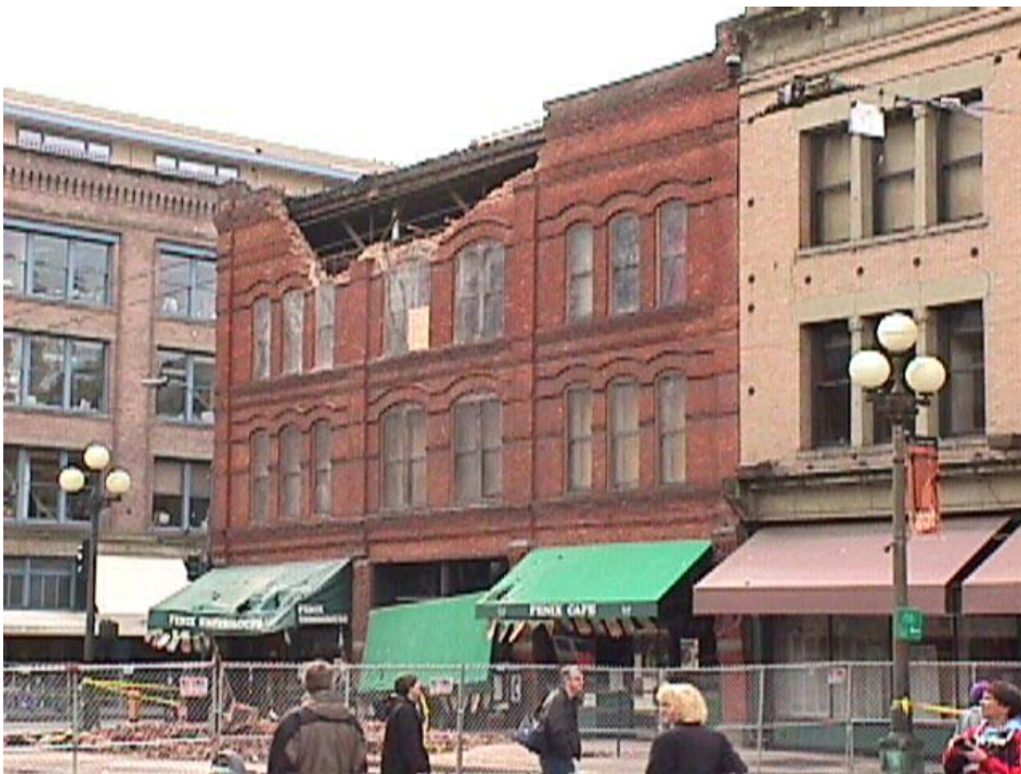
The magnitude 6.8 Nisqually earthquake in 2001 caused serious damage to many older buildings in Seattle's historic Pioneer Square.
