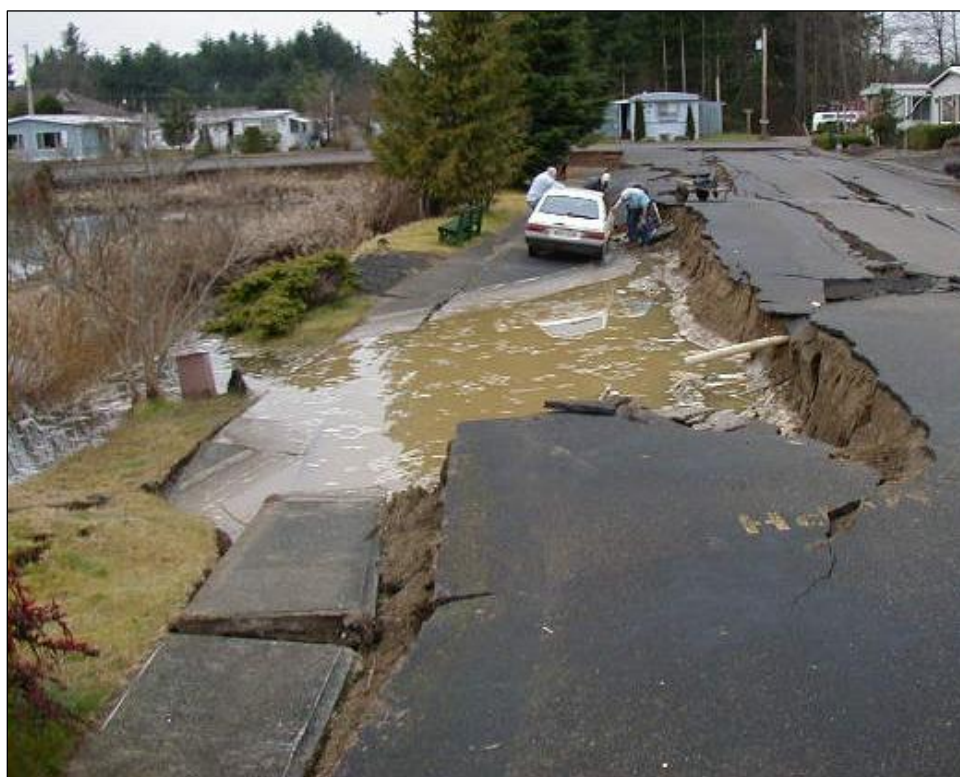
Figure 2. This road failure at Sunset Lake in Tumwater, Washington was caused by the M6.8 Nisqually earthquake in 2001. (Photo: Steven Kramer, University of Washington)
